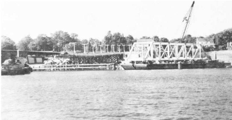
City of Charlevoix temporary bridge, during construction of present day draw bridge, 1947.
